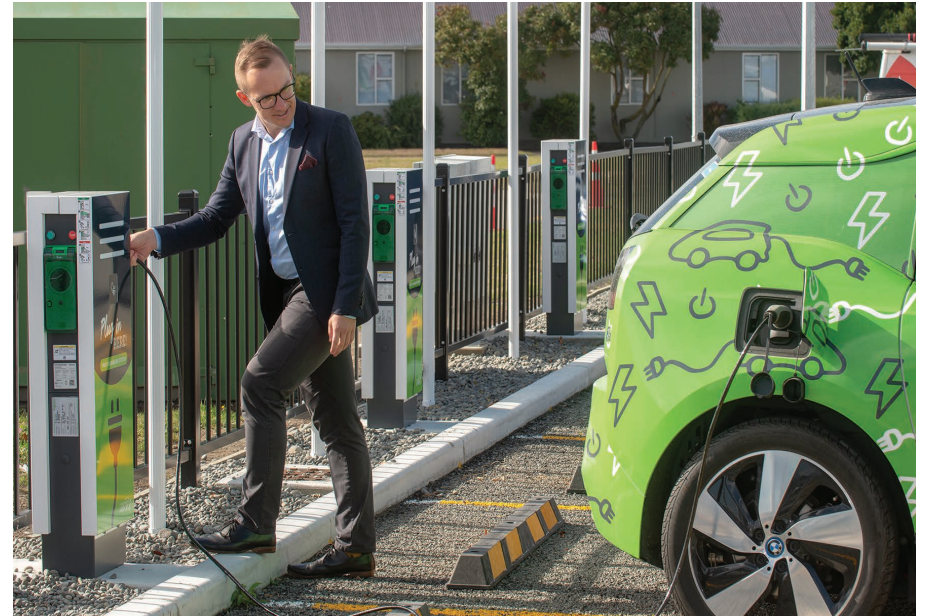
Electric vehicle charging station at Christchurch Airport.
